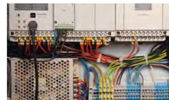
Switch boxes, incl. PLC, for automation purposes
